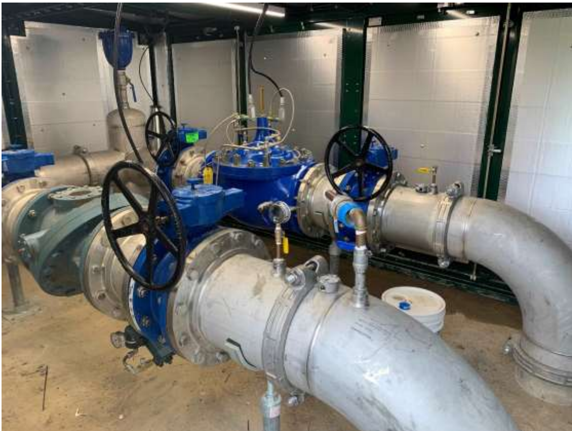
IMAGE | WATER INFRASTRUCTURE AT THE RESERVOIR SITE.
