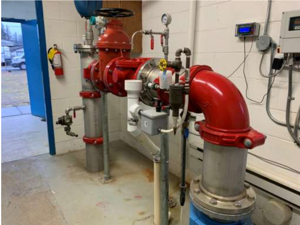
IMAGE | INSIDE THE PUMP HOUSE SHOWING THE WATER MANIFOLD WITH SAMPLE STATION.
